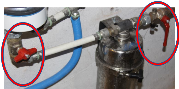
Valves upstream-downstream of the Biofilter
